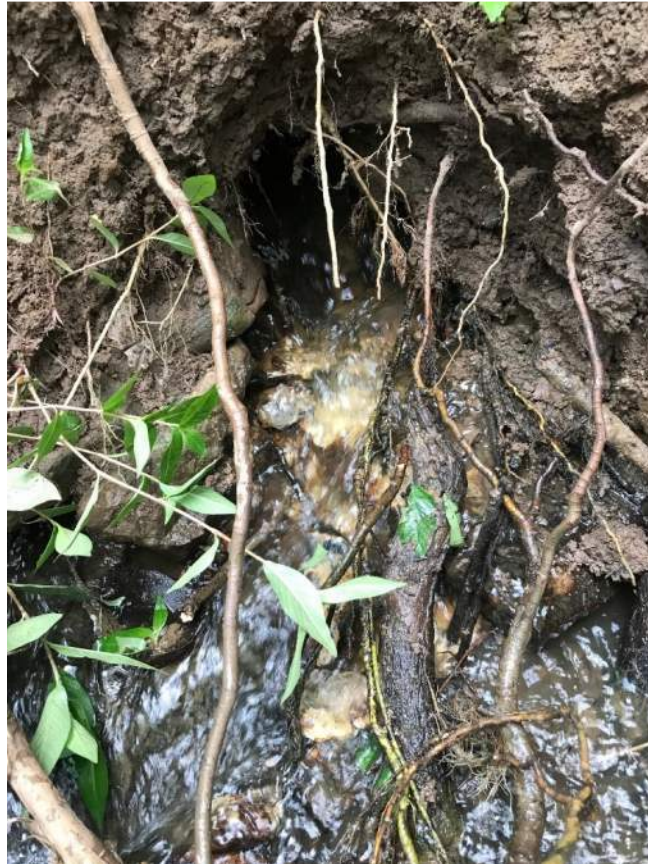
Photo No. 23: Seepage to left of spillway.
