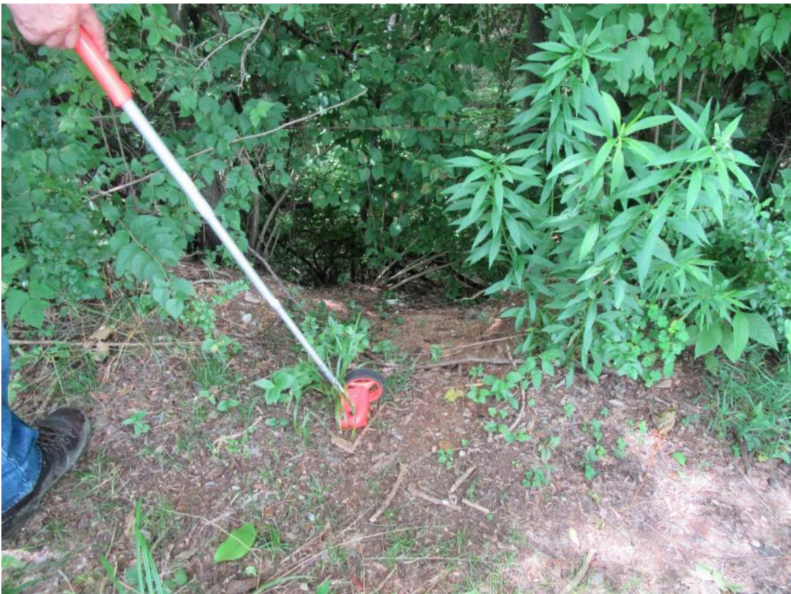
Photo No. 4: Erosion on crest due to possible overtopping.
