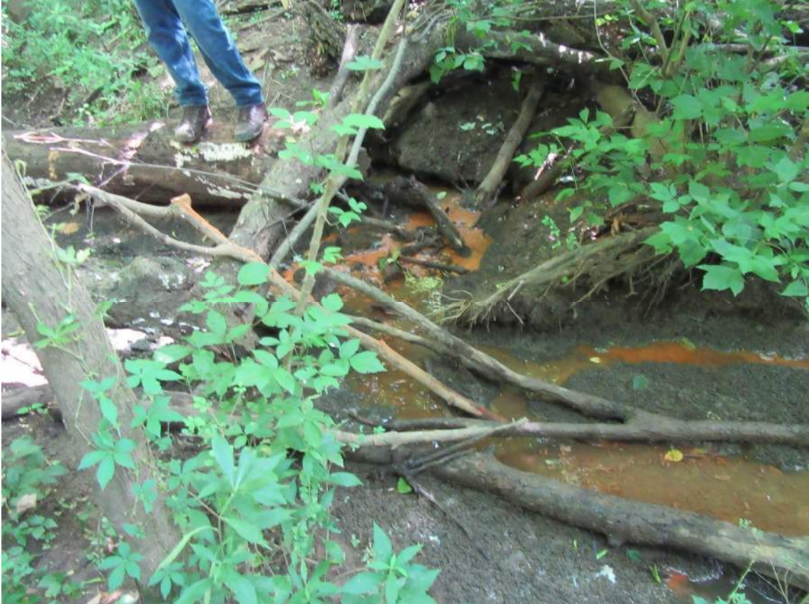
Photo No. 15: Seepage downstream of RCP pipe.
