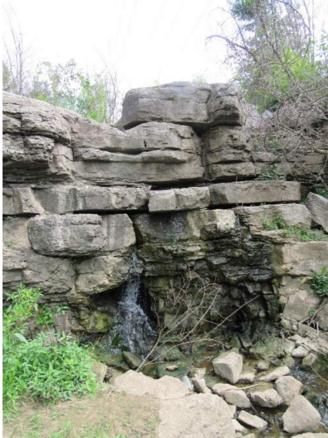
Photo No. 21: Seepage through bedrock at downstream end of spillway discharge channel.
