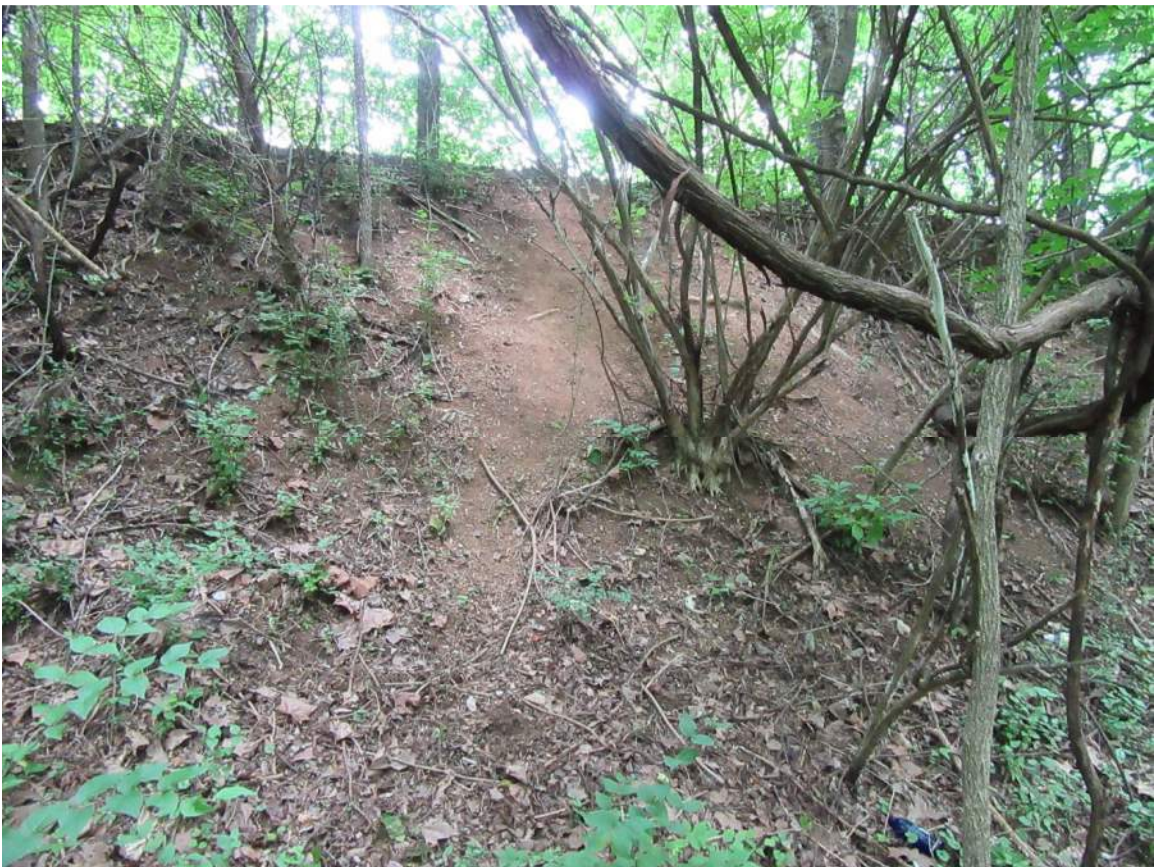
Photo No. 12: Erosion on downstream slope due to possible overtopping.
