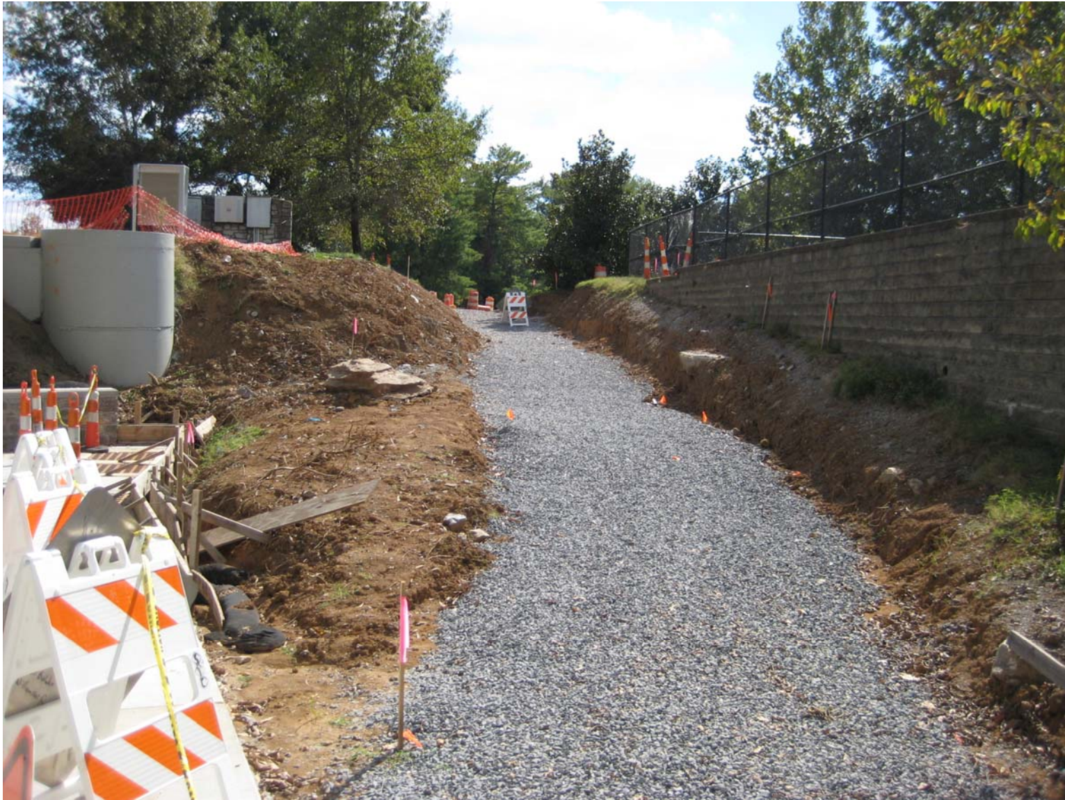
Looking South at Base Stone for ADA-Compliant Ramp Connecting Tunnels and Hunters Bend Elementary School
