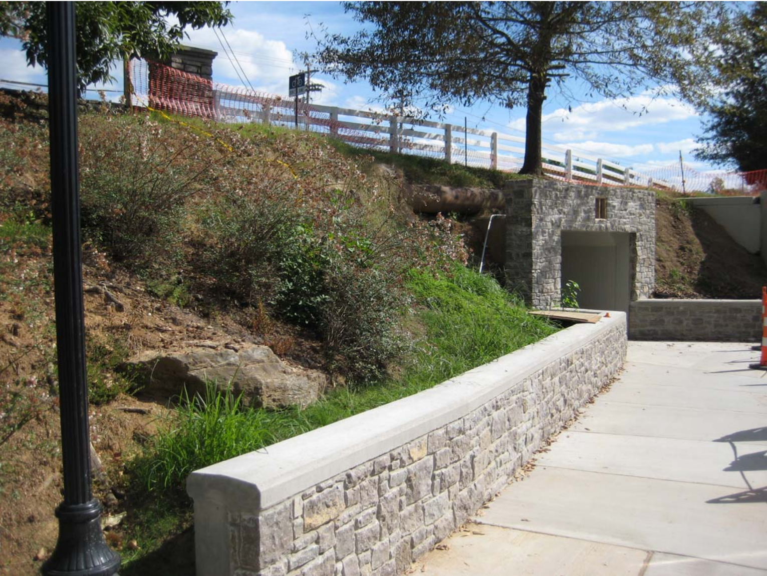
Looking Southeast at Recently Completed Retaining/Sitting Walls and Hillsboro Road Tunnel Surround
