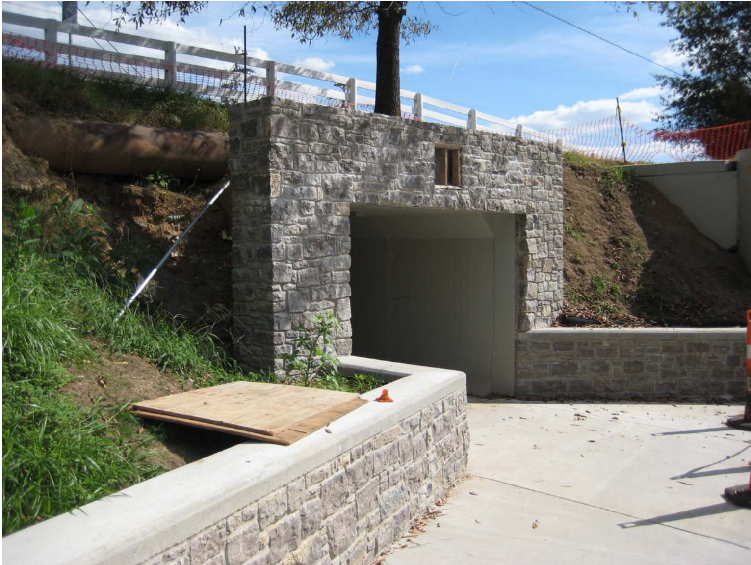
Looking Southeast at Recently Completed Hillsboro Road Tunnel Surround and Small Retaining/Sitting Walls
