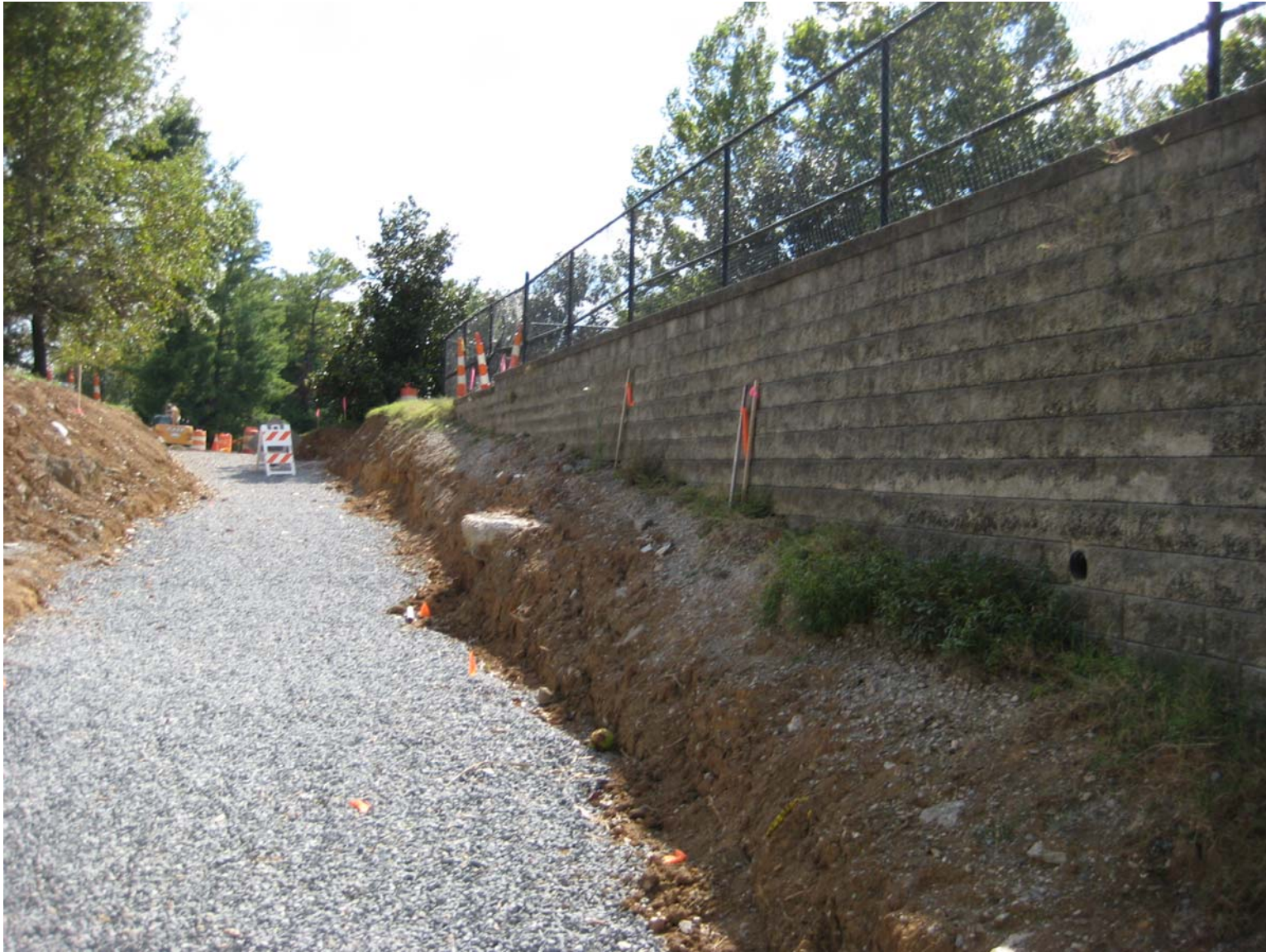
Existing, Private Property (Daycare) Retaining Wall Directly Adjacent to West Side of Proposed ADA-Compliant Ramp
