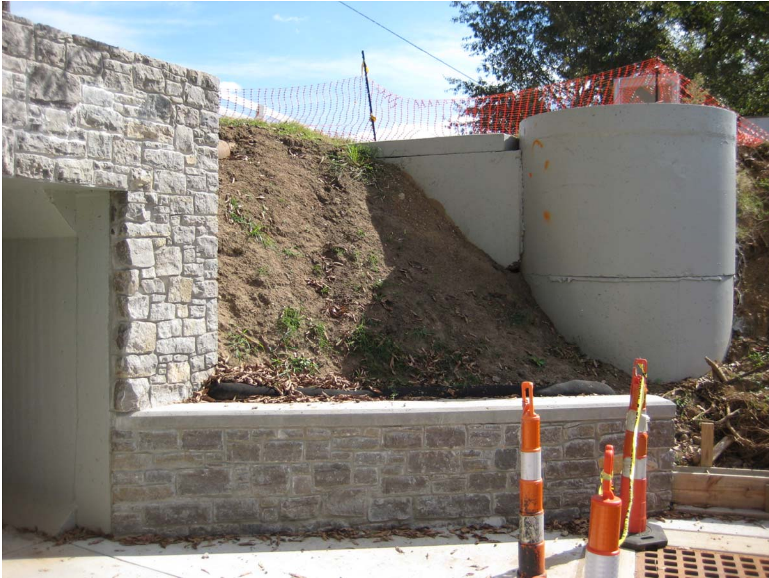
Looking Southeast at Steep Slope between Hillsboro Road Tunnel and Pump Manhole
