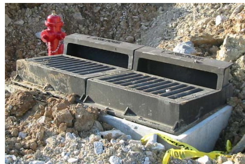
Vane grate for curb and gutter section
