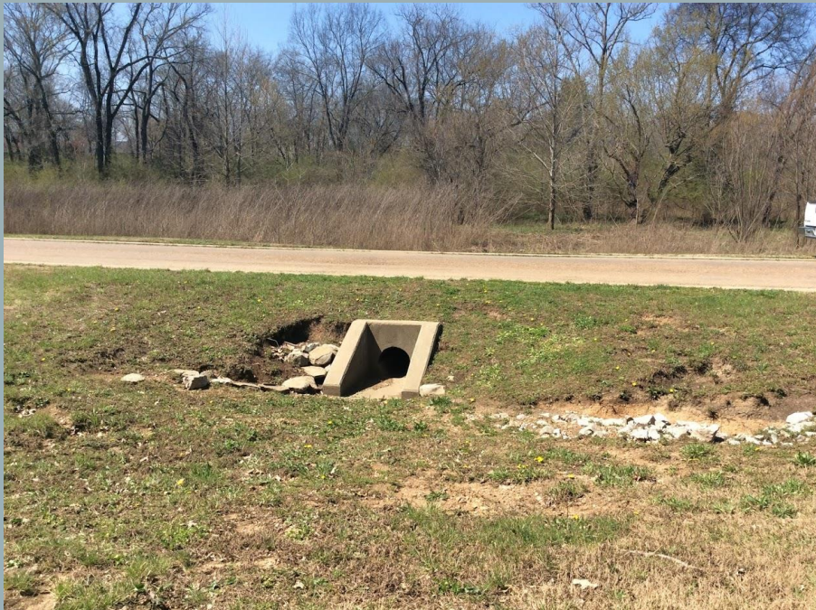
Eastern Flank: Fix erosion draining to stream
